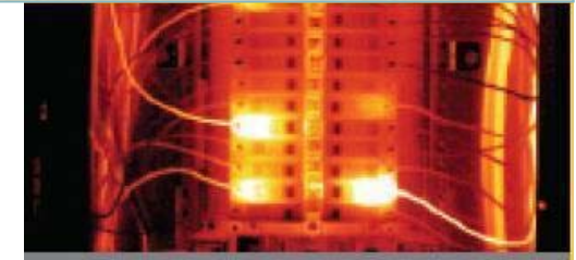
Circuit Breaker Problems
